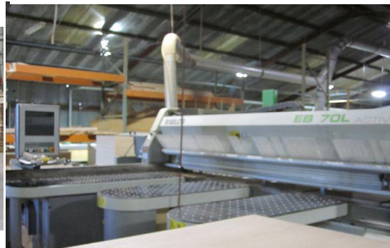
One of the panel saws.
